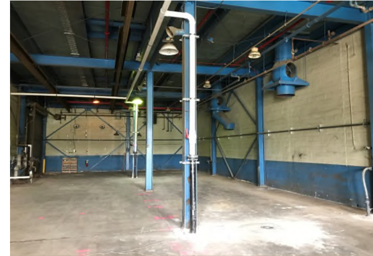
Industrial building with active vapor mitigation system
