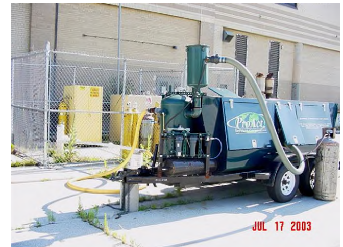
ICE pilot system at DSCP, image courtesy of Tetra Tech
